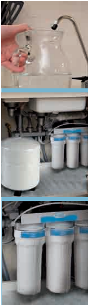
UNDER SINK - R.O. SYSTEM
